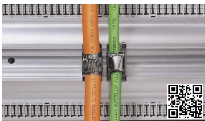
EMC safety inside the control cabinet
